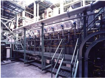
Carbonizing furnace system
