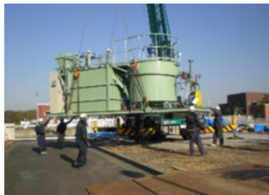
High-rate coagulation settling unit
