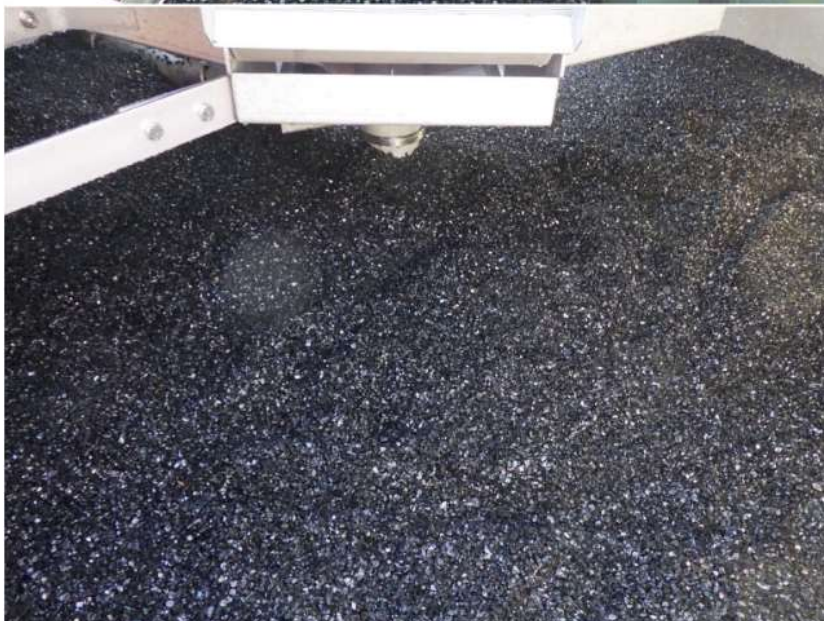
Photo 3: Inside of biofilm filtration tank filled with carrier
