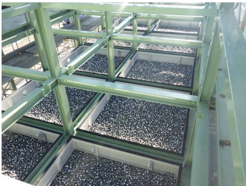
Photo 2: Inside of DHS filter bed filled with carrier
