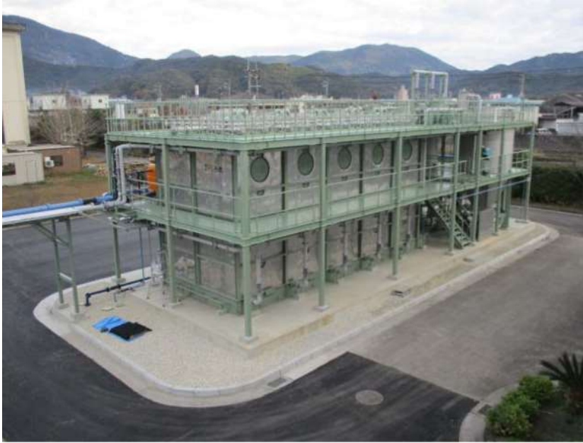
Photo 1: Appearance of demonstration facilities (left:DHS filter bed, right:biofilm filtration tank)
