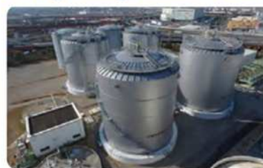
Steel digestion tank
