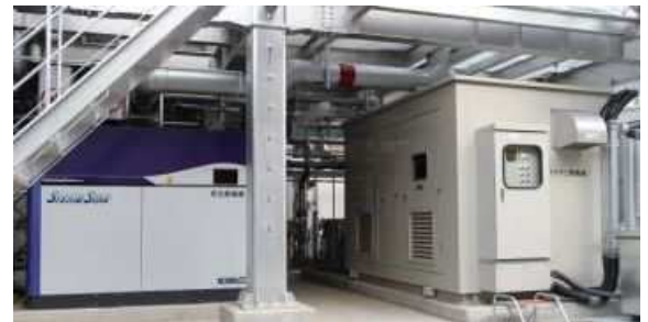
Left: Screw type generator Right: Binary type generator
