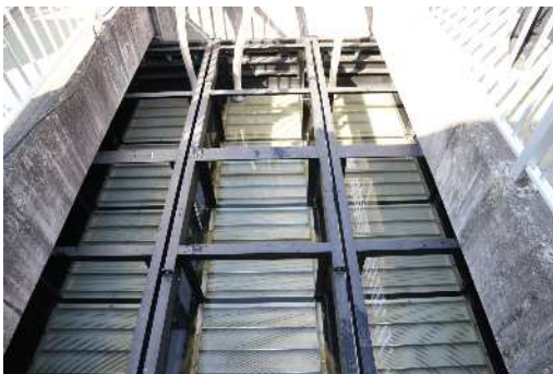
The upper part of filtration area
