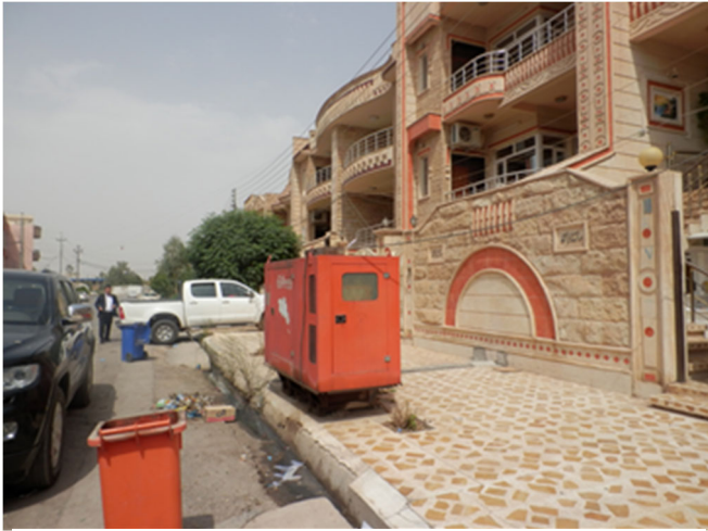
Photo 3: Home standby generator
