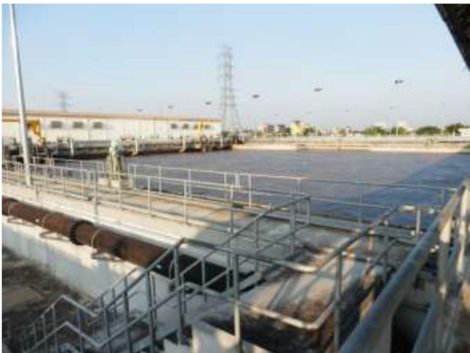
Photo 3: WWTP using activated sludge process
