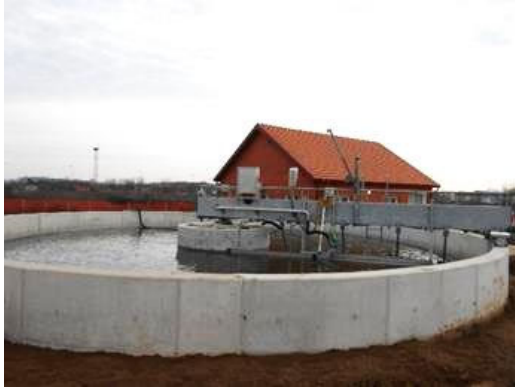
Primary settling tank (A building of water quality lab in the back)
