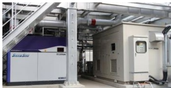
Left: Screw type generator Right: Binary type generator
