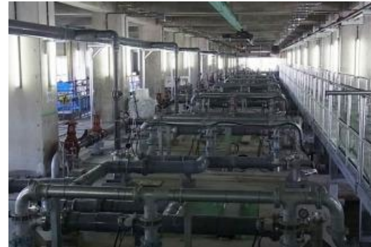
The upper side of the high-rate carrier filling bed
