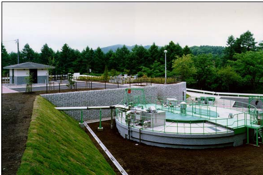
Nobeyama Wastewater Treatment Plant (Minanimaki-village, Nagano Prefecture)
