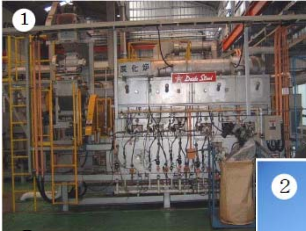
① Development of Carbonization system for sewage sludge fuelization
