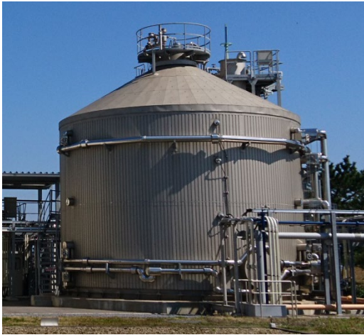
Non-powered stirring type digestion tank
